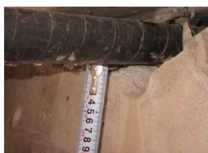
②A2橋台：沈下(50mm)
